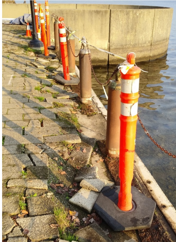
Plaza damage around Handsome Bollards
