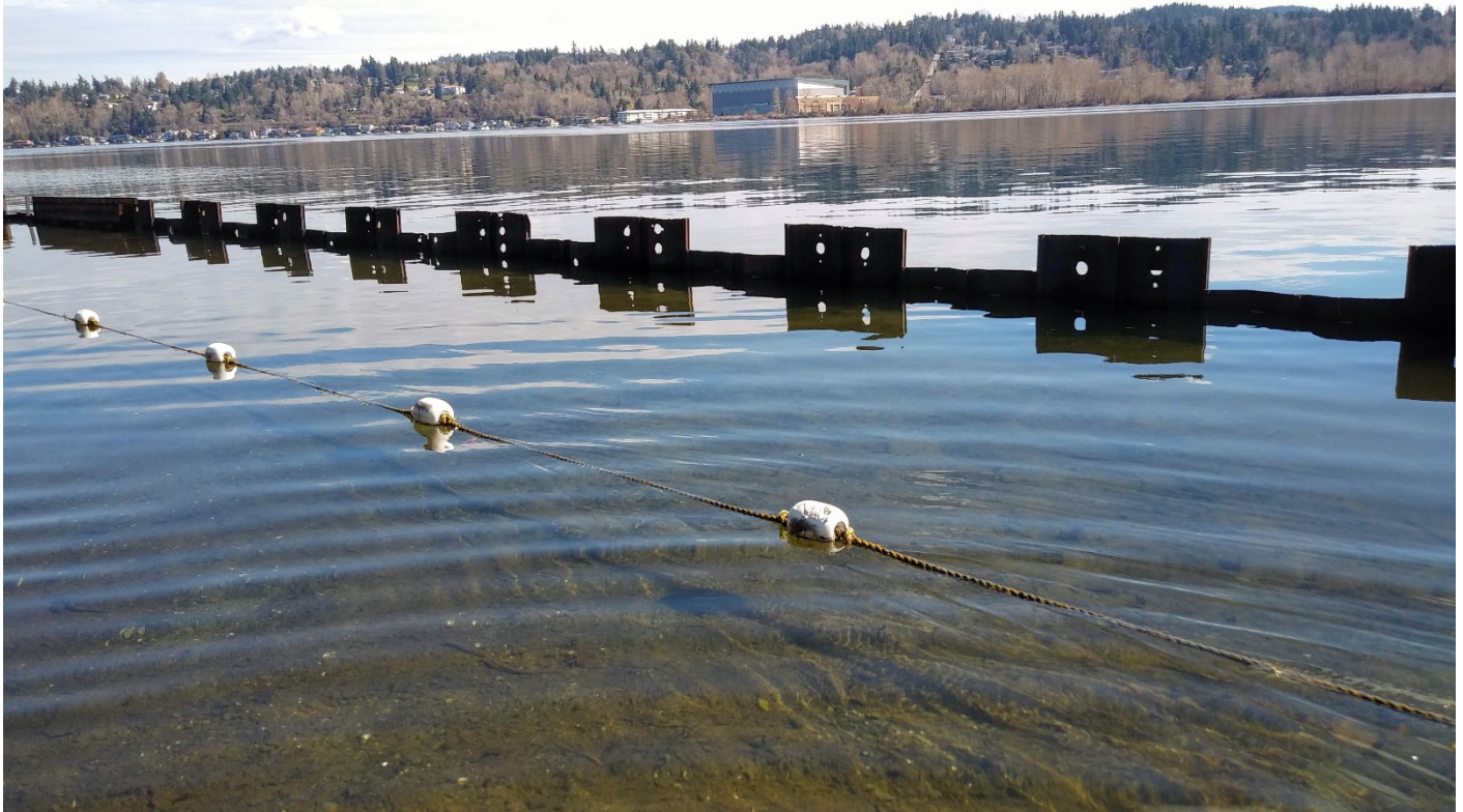
Clarke Beach swim enclosure showing the swim float line and sheet piles missing the wooden cap rail
