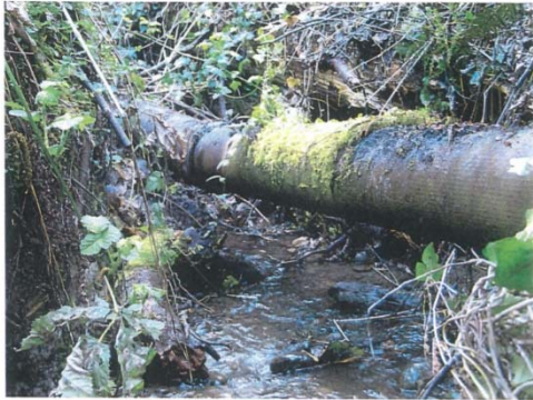
Exposed sewer line in watercourse (before)
