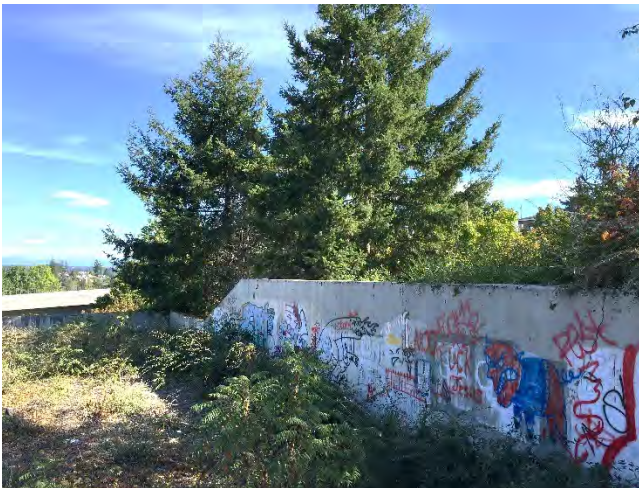
WSDOT maintenance building rooftop – walls with graffiti.
