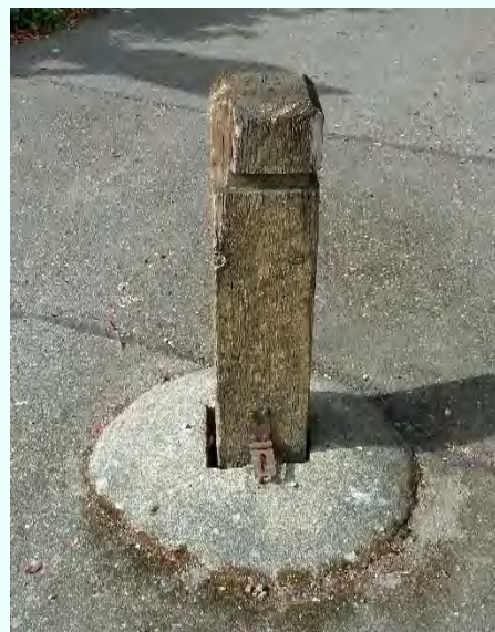
Removable bollard (#60) in the center position of a group of bollards.
