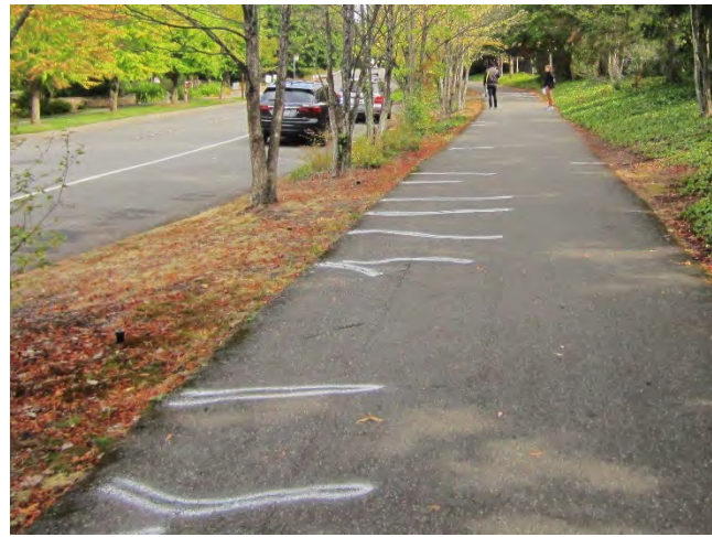
Heaving paving is a potential hazard for trail users.
