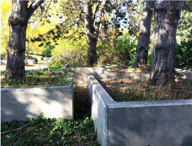
Overgrown trees in landscape planters.
