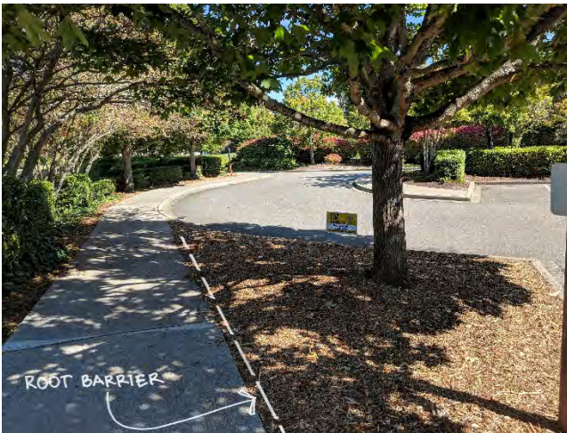
Trench along paving edge to stop tree roots from heaving adjacent paving. Install 18" depth root barrier to prevent future root problems.
