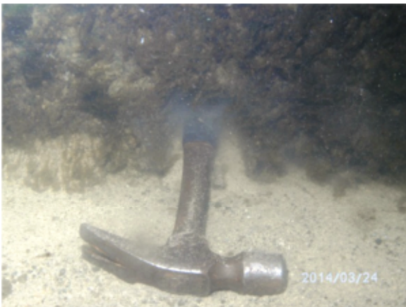
Photo 5C – Undermined bulkhead toe
