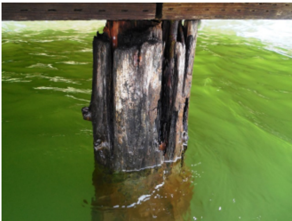
Photo 21C – Severely decayed pile
