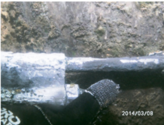
Photo 21A – Stripped / corroded connector
