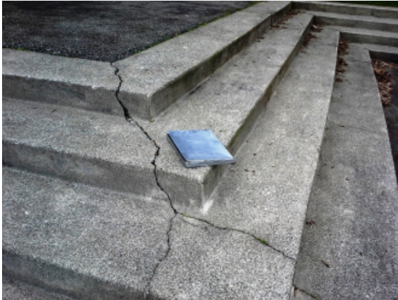
Photo 7B – Cracked shoreline steps
