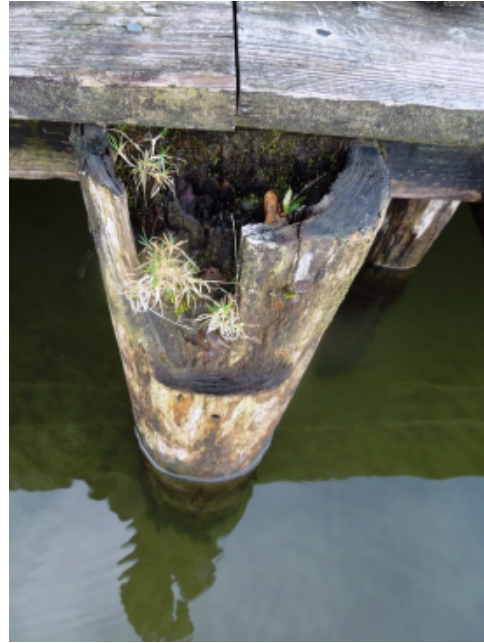
Photo 32C – Decayed pile, small pier
