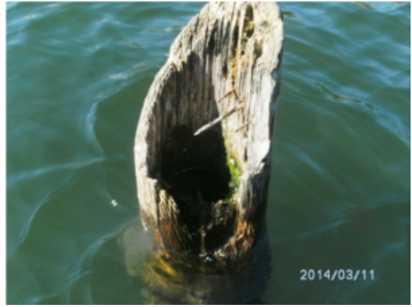
Photo 26A – Deteriorated mooring pile
