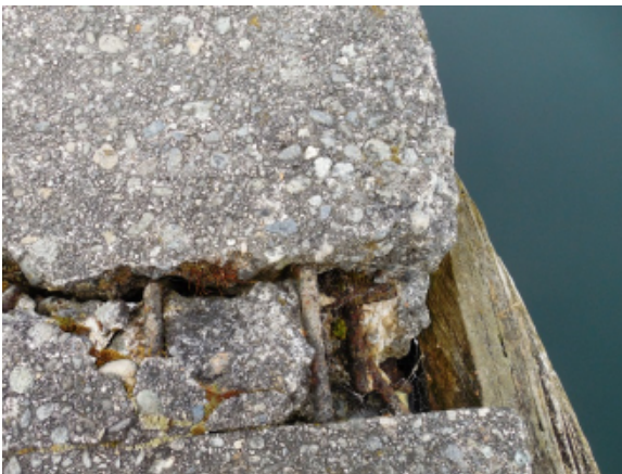
Photo 9A – Deteriorated pier slab
