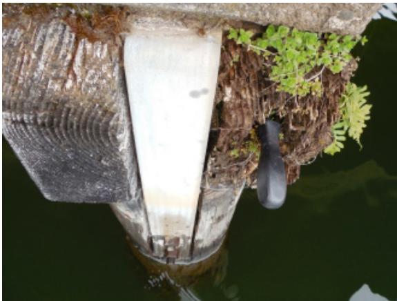
Photo 15A – Deteriorated cap beam end
