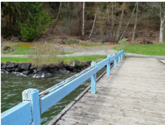
Photo 11B – Deteriorated wood rail
