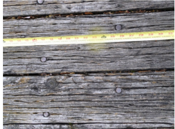
Photo 14B – Weathered wood decking
