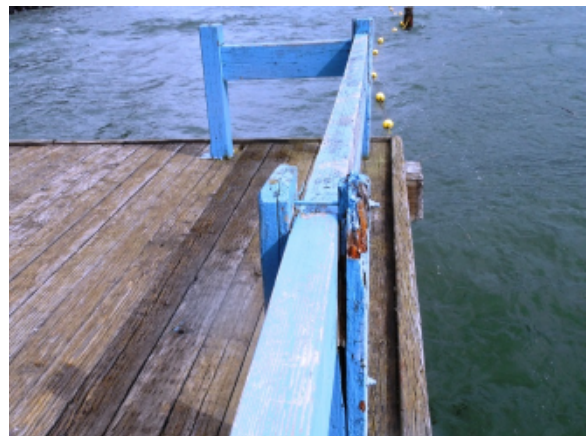
Photo 12B – Deteriorated wood rail
