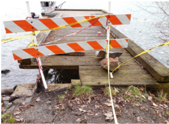
Photo 21B – Fire damage at small pier
