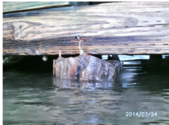
Photo 22C – Severely decayed pile, loss of bearing
