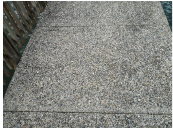
Photo 14C – Cracked concrete pier slab
