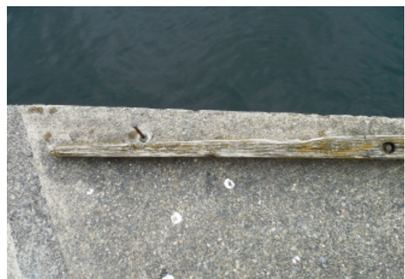
Photo 12A – Deteriorated / loose bull rail
