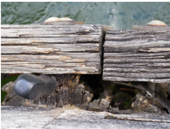
Photo 17C – Decayed top of pile
