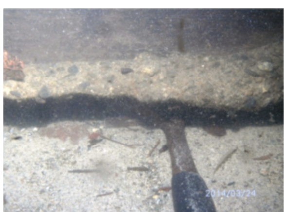
Photo 6C – Undermined bulkhead toe
