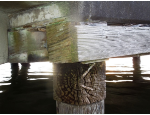
Photo 25A – Deteriorated cap beam (small pier)
