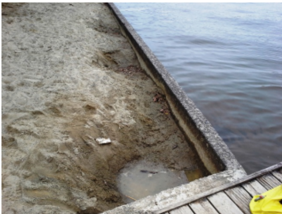
Photo 3C – Eroded sand, Beach 1
