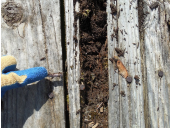
Photo 31C – Decayed decking, small pier
