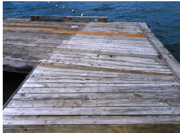
Photo 30C – Small pier decking, past repair
