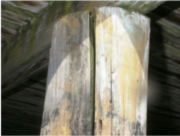
Photo 19B – Split pile
