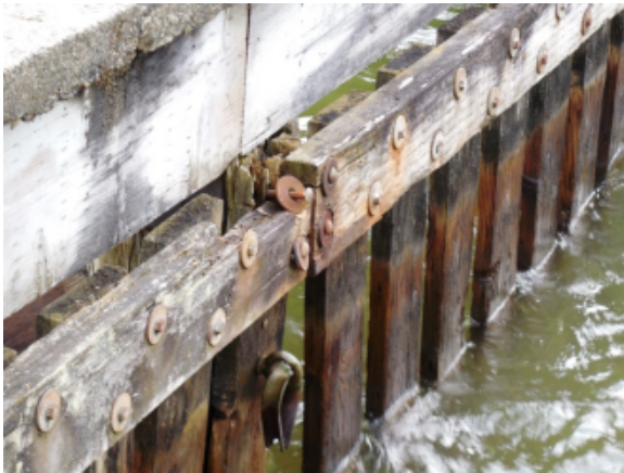
Photo 13C – Deteriorated skirt wall
