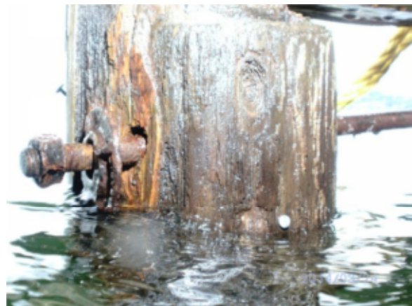
Photo 24C – Decayed pile, loose connection hardware
