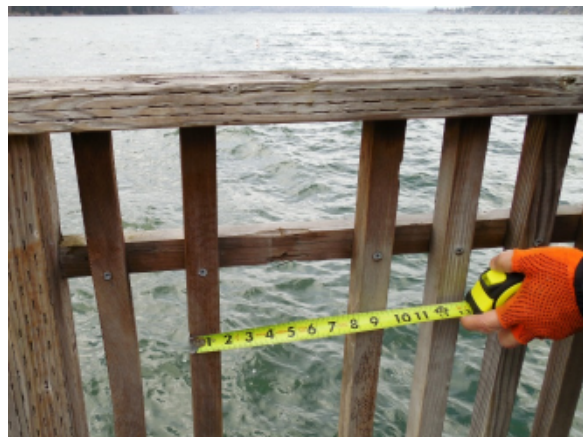
Photo 12C – Missing rail picket
