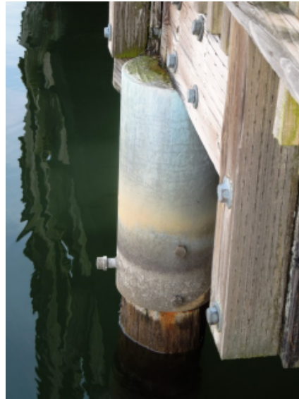
Photo 20C – “Canned” pile (previous repair)
