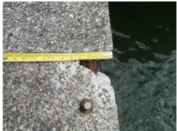
Photo 16C – Weathered, spalled slab
