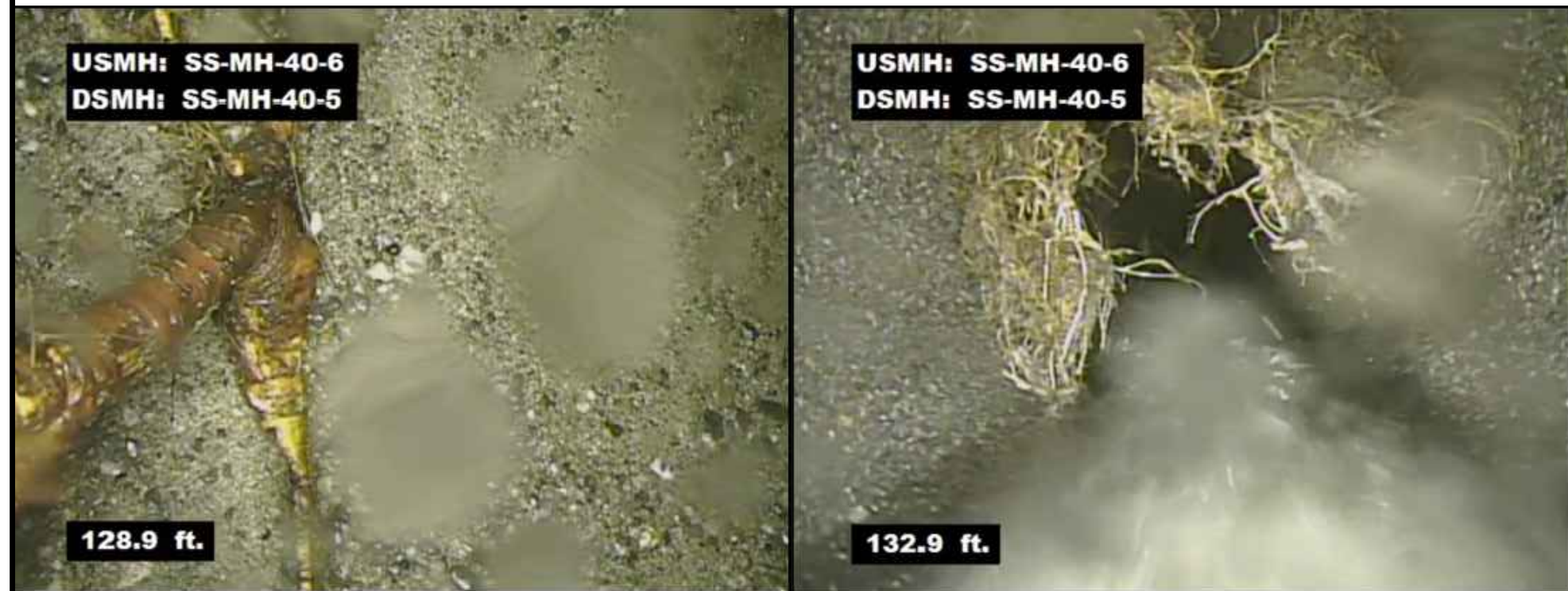
EXISTING MAINLINE CONDITIONS AT SELECT LOCATIONS: MH 5 TO MH 6
