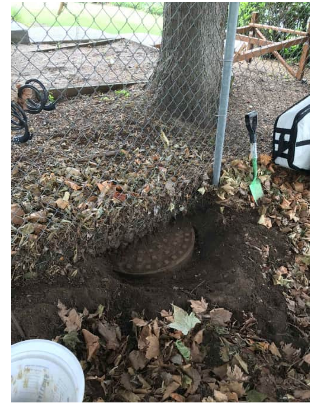
MH LID ACCESS AT SELECT LOCATION: MH 40-2.1
