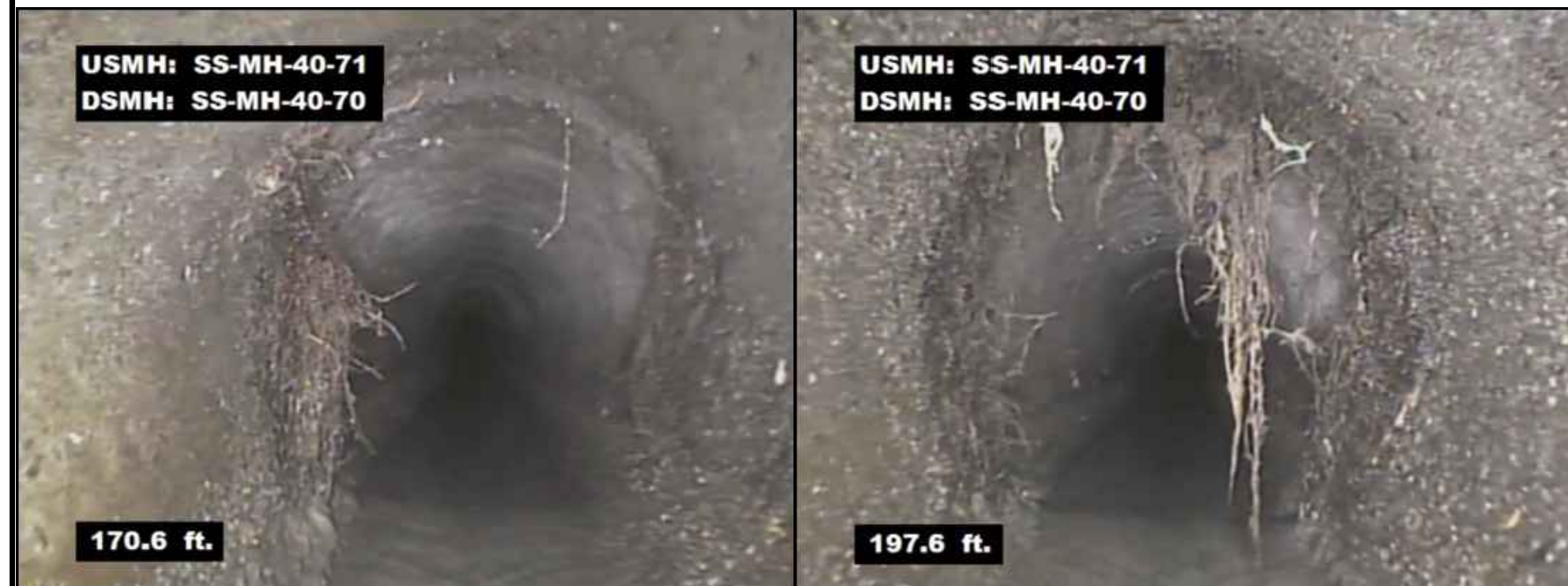
EXISTING MAINLINE CONDITIONS AT SELECT LOCATIONS: MH 71 TO MH 70
