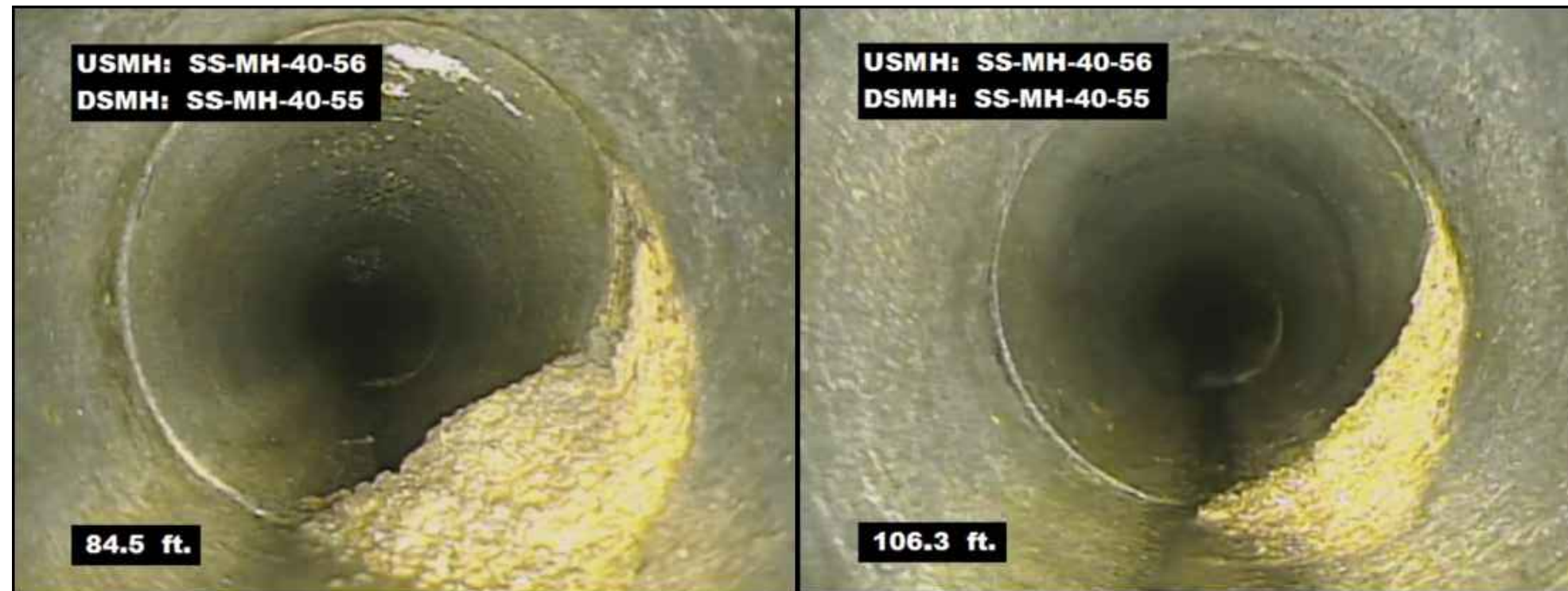
EXISTING MAINLINE CONDITIONS AT SELECT LOCATIONS: MH 56 TO MH 55
