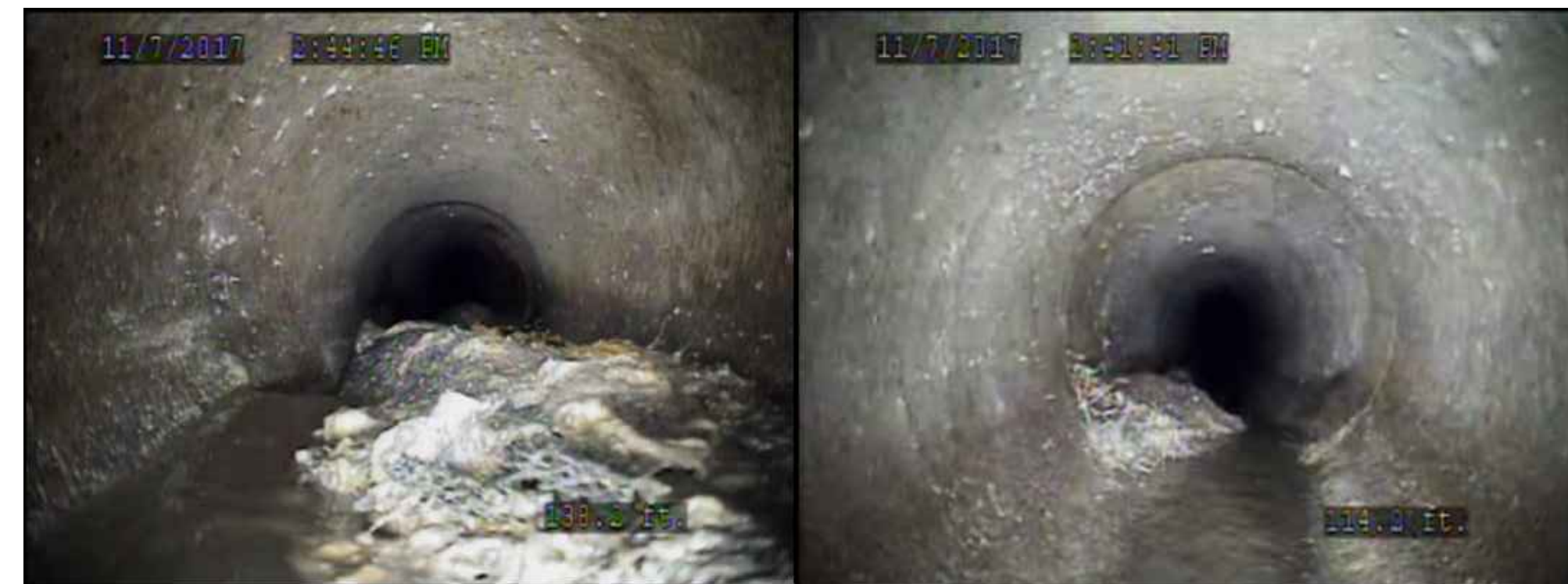
EXISTING MAINLINE CONDITIONS AT SELECT LOCATIONS: MH 82 TO MH 81
