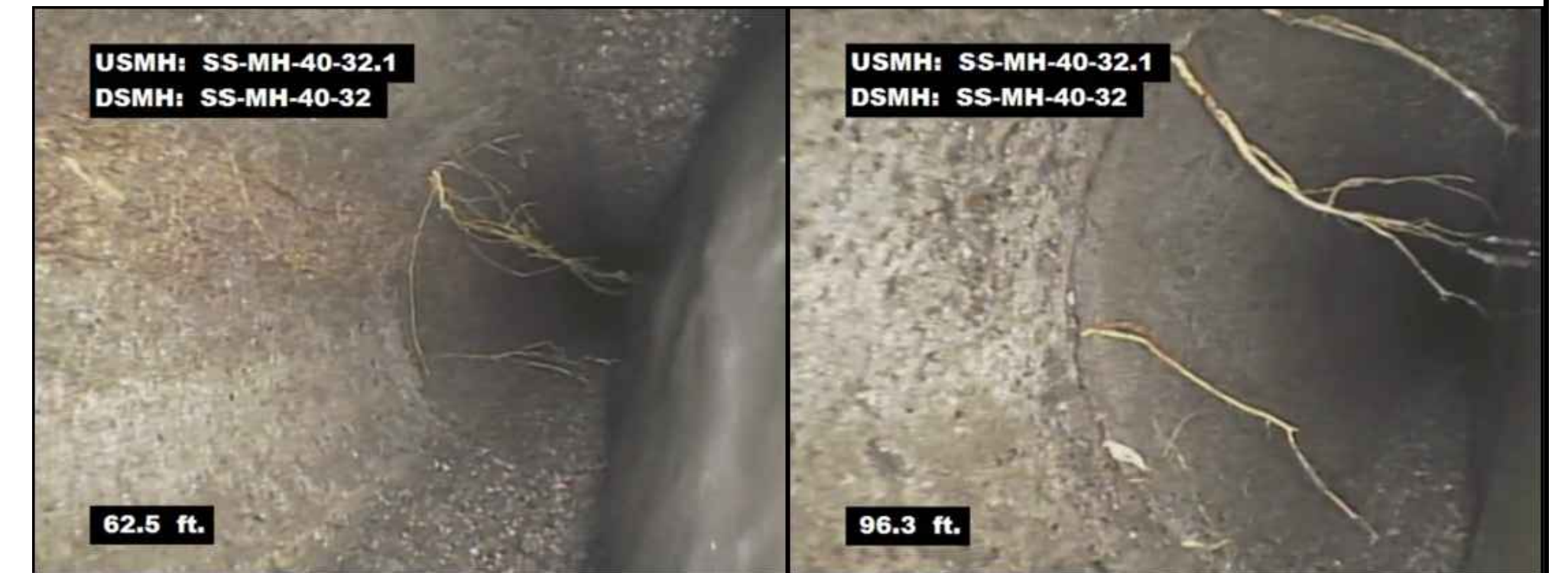
EXISTING MAINLINE CONDITIONS AT SELECT LOCATIONS: MH 32.1 TO MH 32
