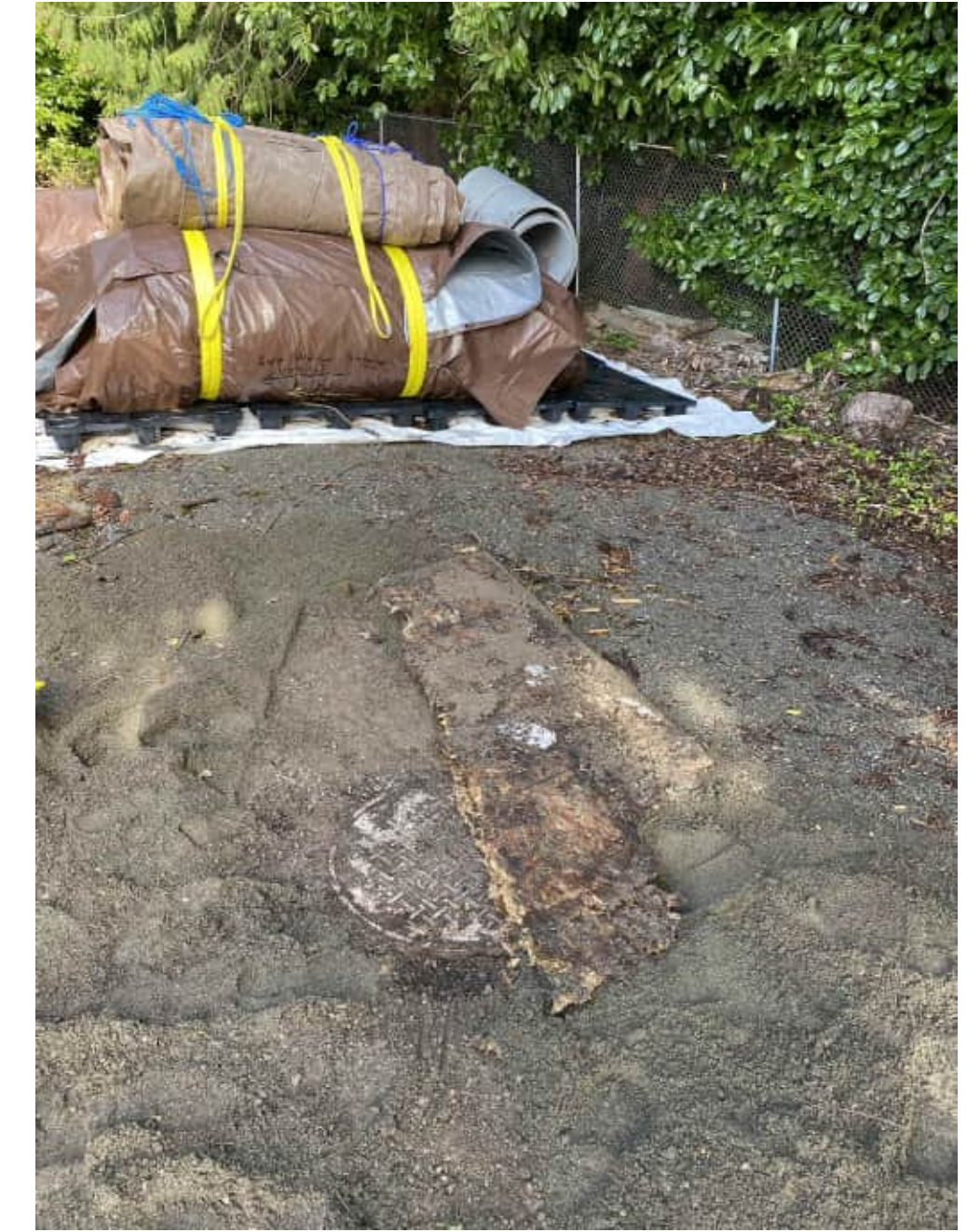
MH LID ACCESS AT SELECT LOCATION: MH 40-5 (1)
