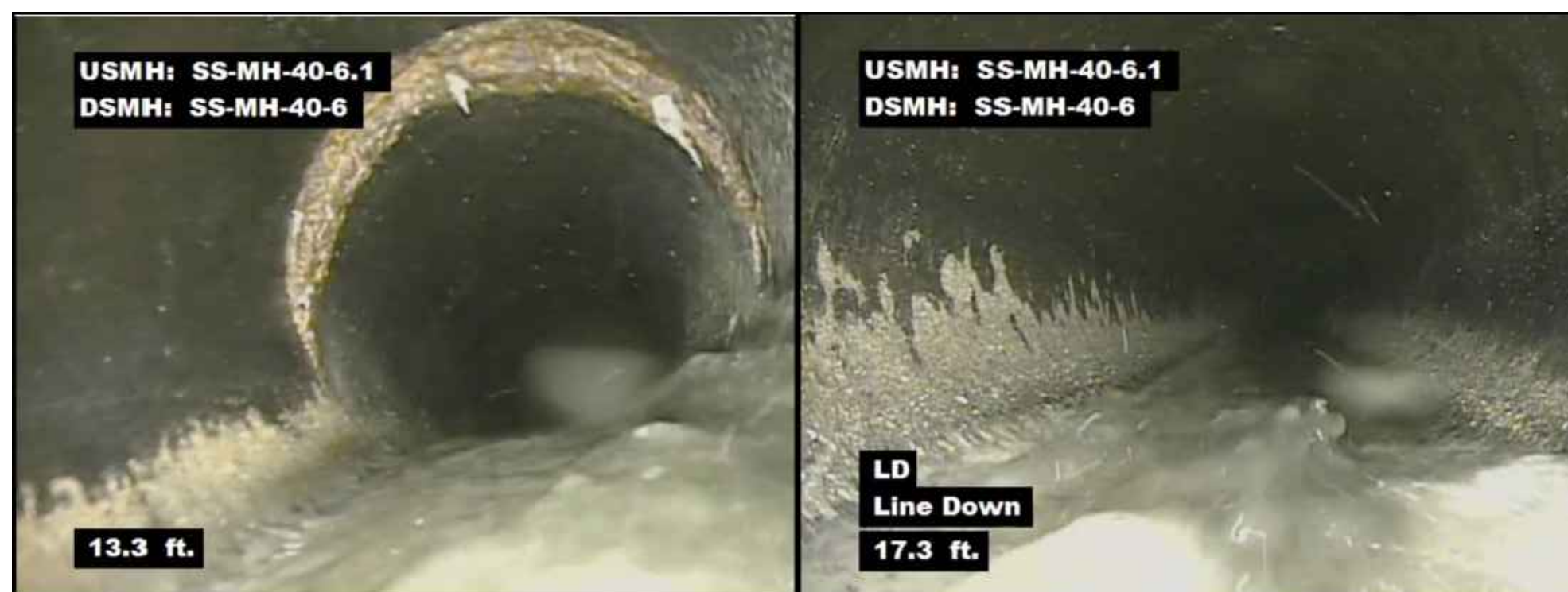
EXISTING MAINLINE CONDITIONS AT SELECT LOCATIONS: MH 6.1 TO MH 6
