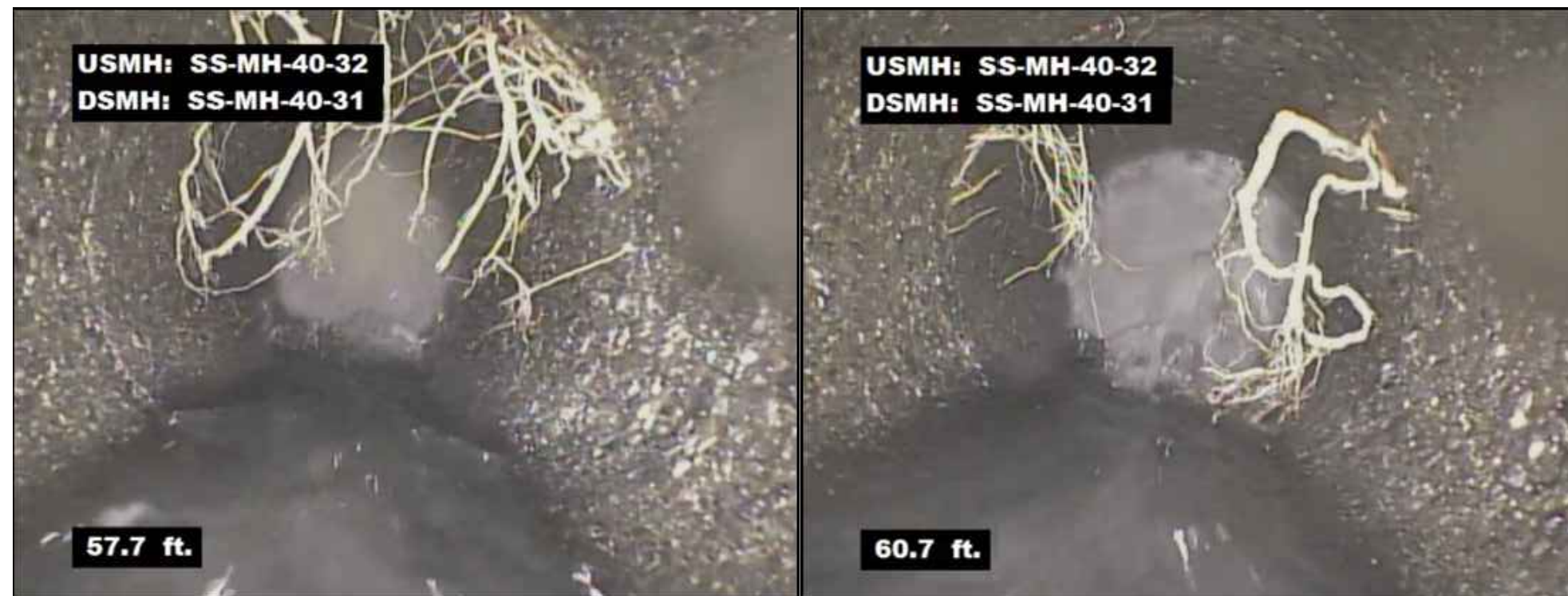
EXISTING MAINLINE CONDITIONS AT SELECT LOCATIONS: MH 32 TO MH 31
