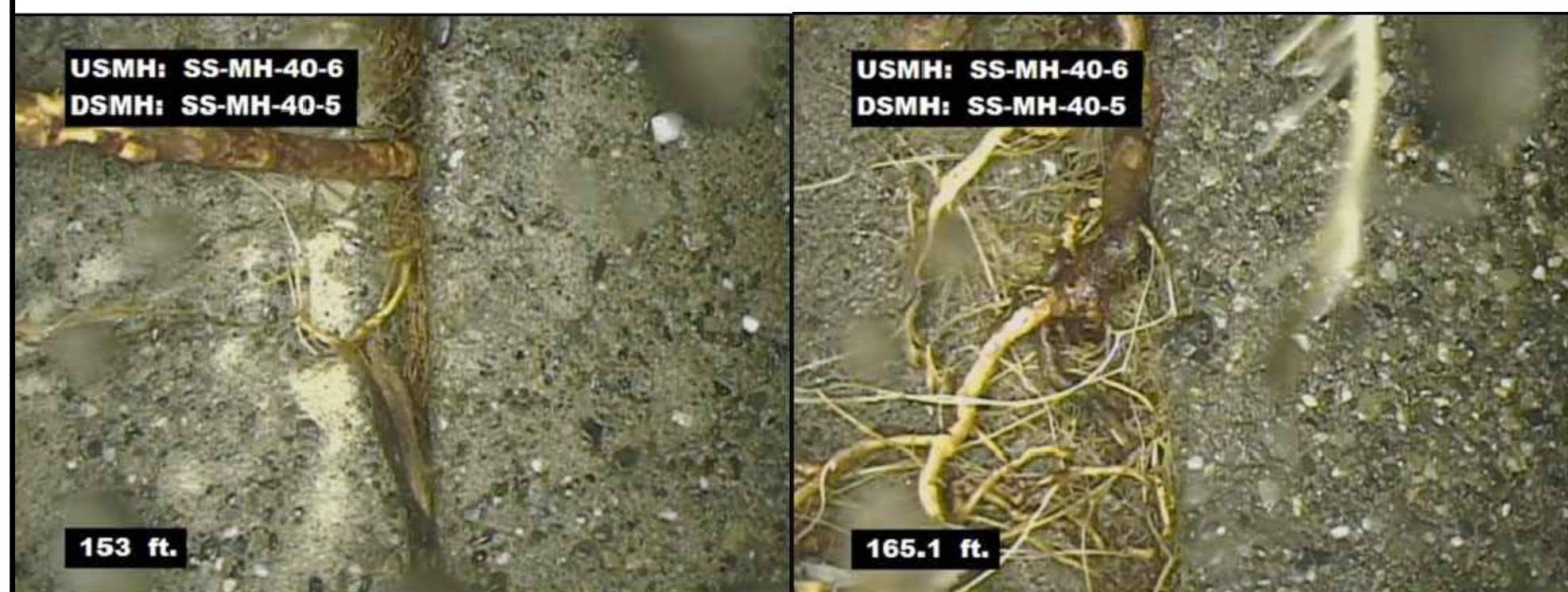
EXISTING MAINLINE CONDITIONS AT SELECT LOCATIONS: MH 5 TO MH 6
