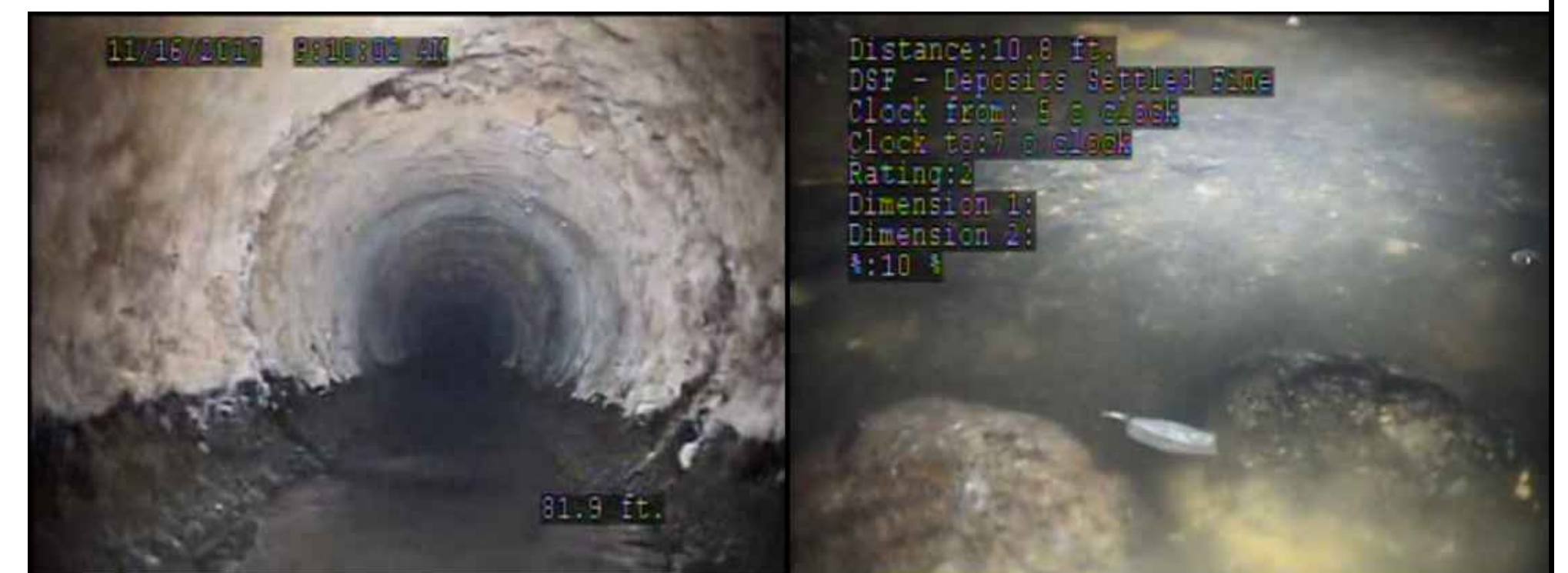
EXISTING MAINLINE CONDITIONS AT SELECT LOCATIONS: MH 68 TO MH 67
