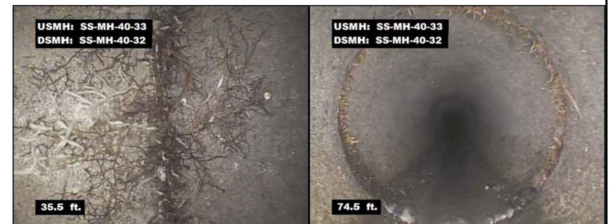
EXISTING MAINLINE CONDITIONS AT SELECT LOCATIONS: MH 33 TO MH 32
