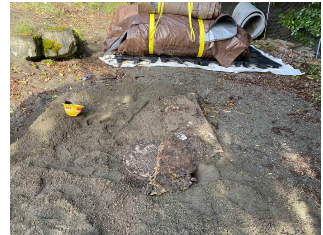
MH LID ACCESS AT SELECT LOCATION: MH 40-5 (2)
