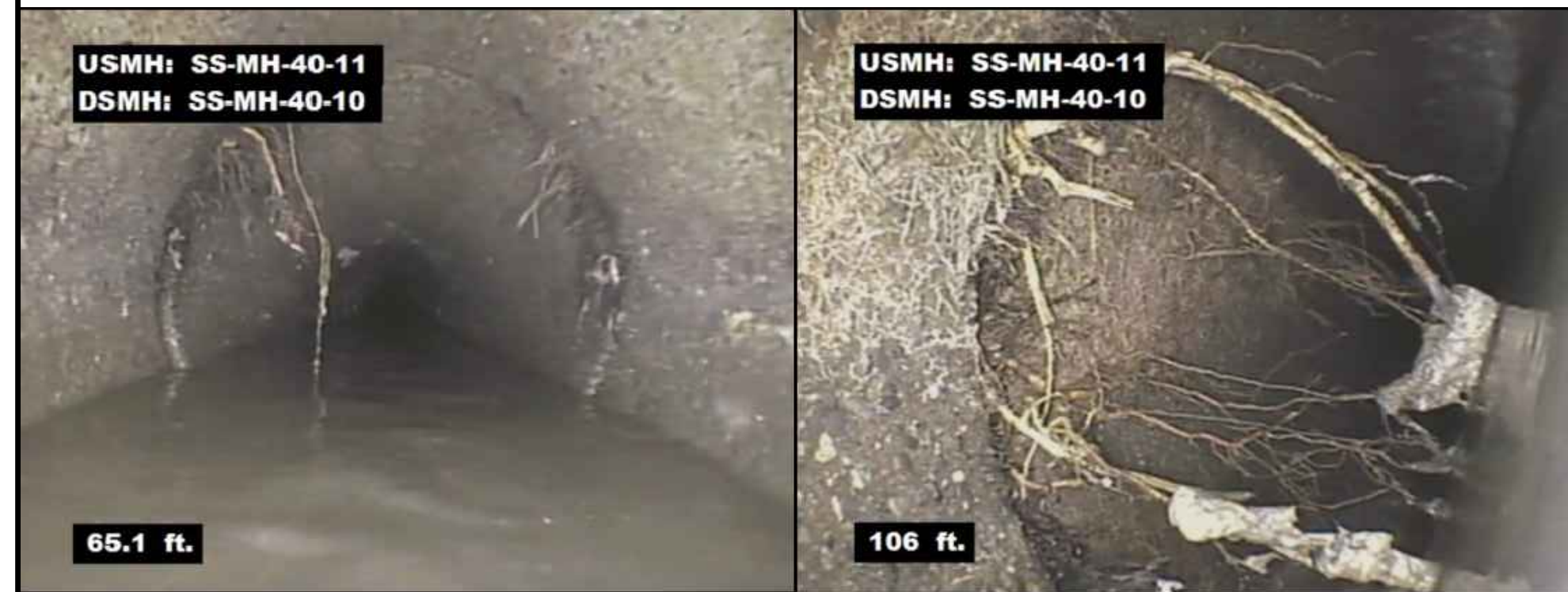
EXISTING MAINLINE CONDITIONS AT SELECT LOCATIONS: MH 11 TO MH 10
