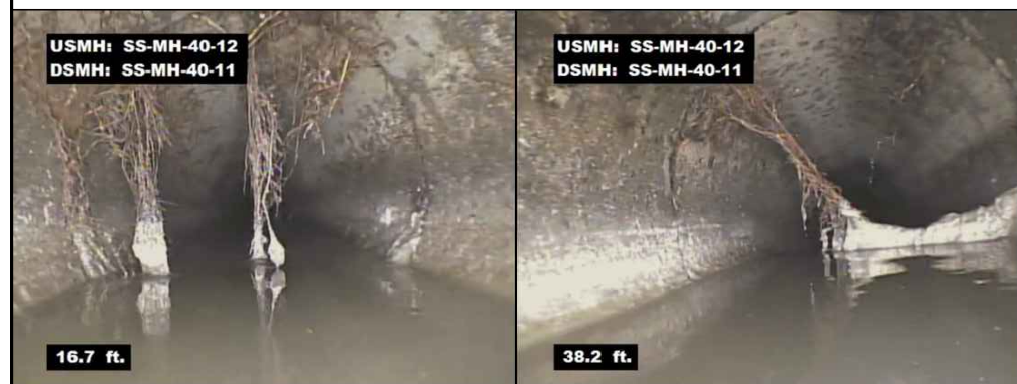
EXISTING MAINLINE CONDITIONS AT SELECT LOCATIONS: MH 12 TO MH 11
