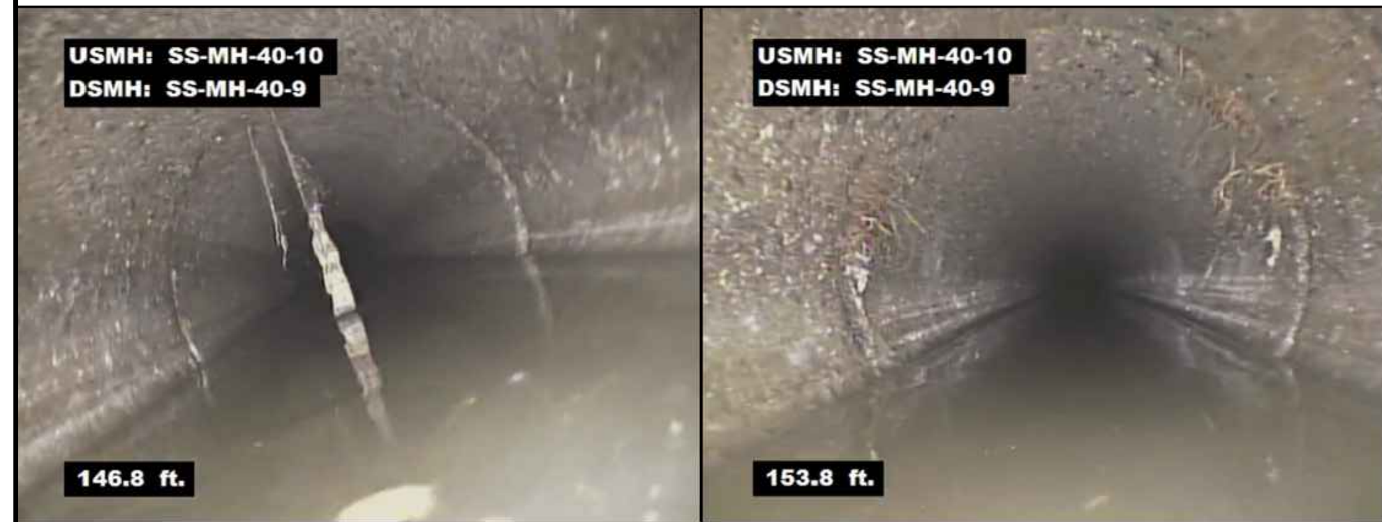
EXISTING MAINLINE CONDITIONS AT SELECT LOCATIONS: MH 10 TO MH 9
