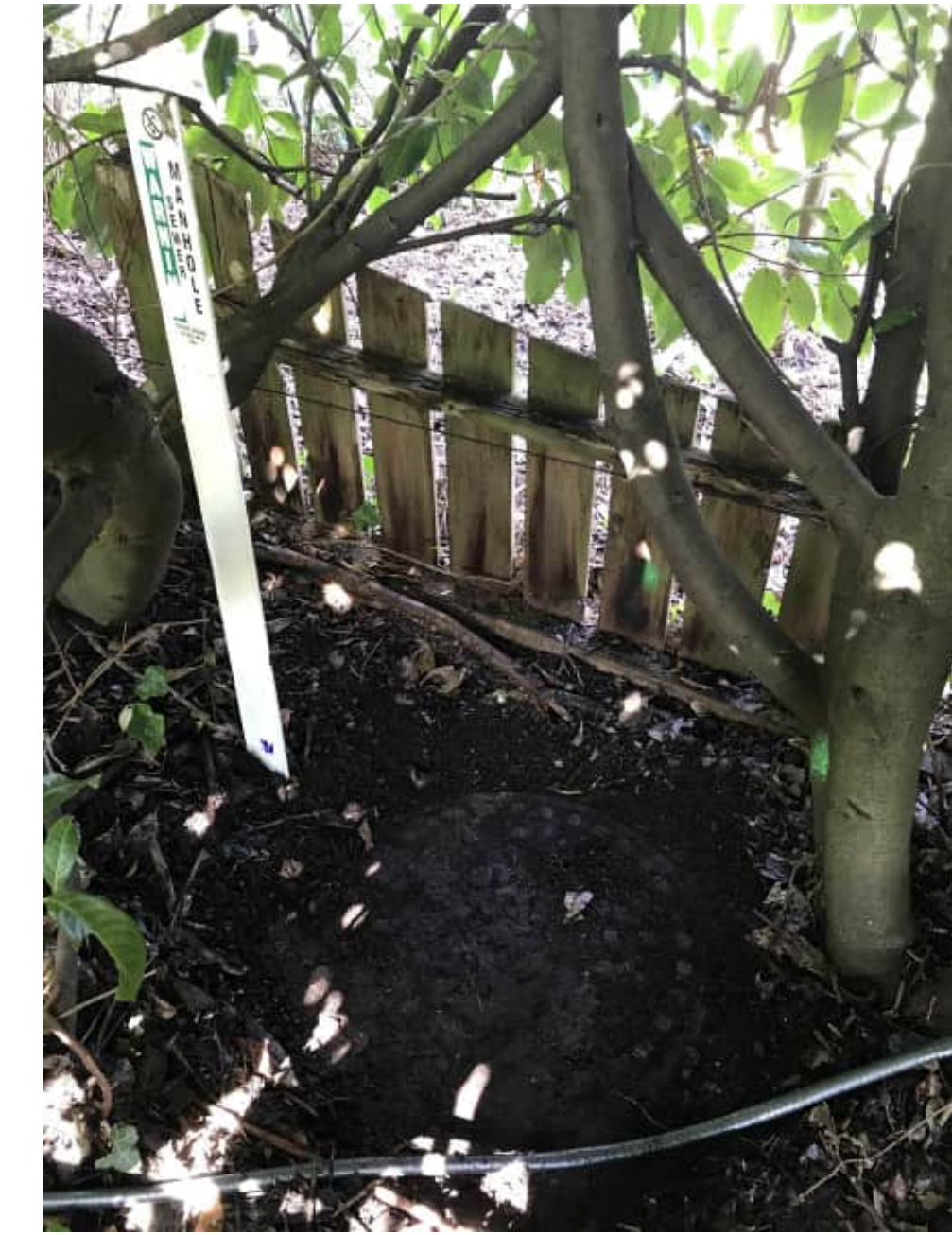
MH LID ACCESS AT SELECT LOCATION: MH 40-953
