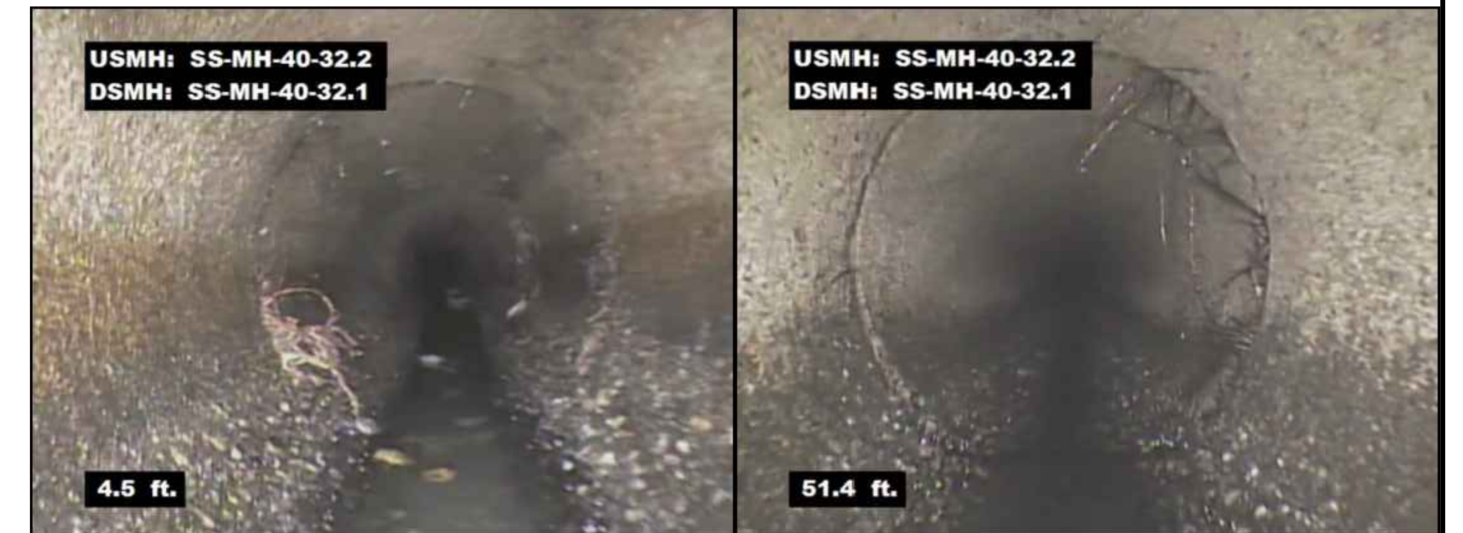
EXISTING MAINLINE CONDITIONS AT SELECT LOCATIONS: MH 32.2 TO MH 32.1
