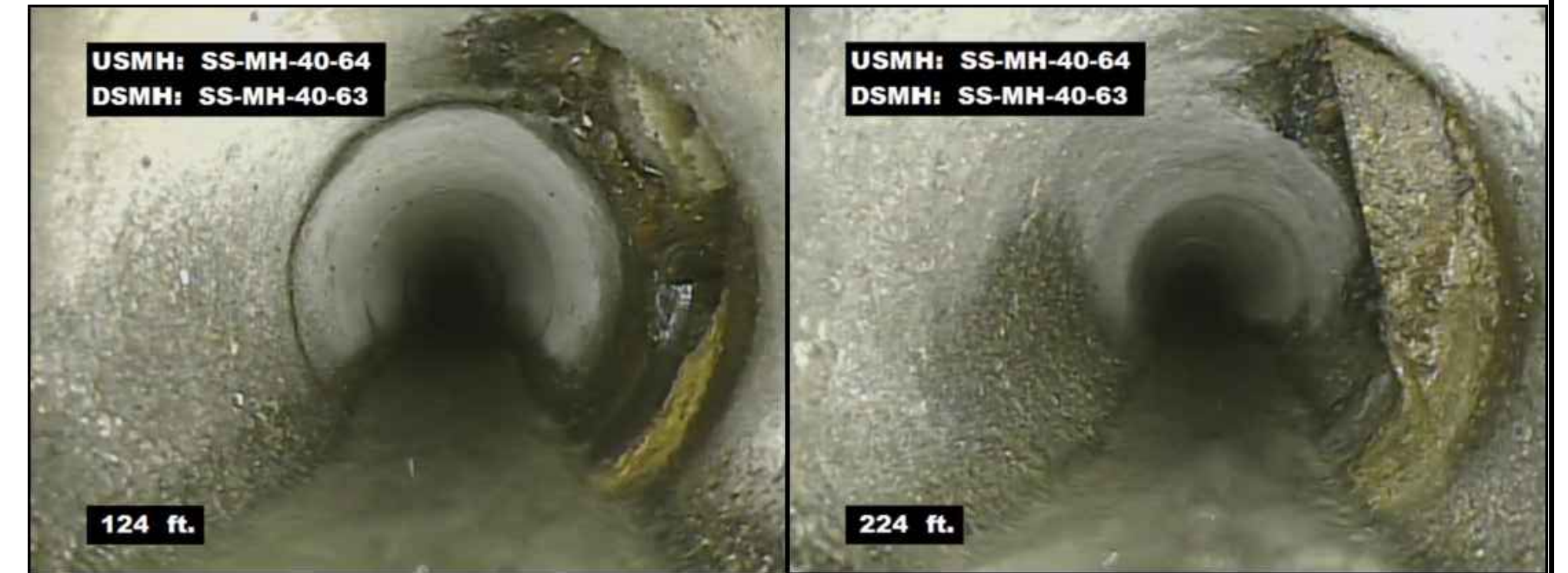
EXISTING MAINLINE CONDITIONS AT SELECT LOCATIONS: MH 64 TO MH 63
