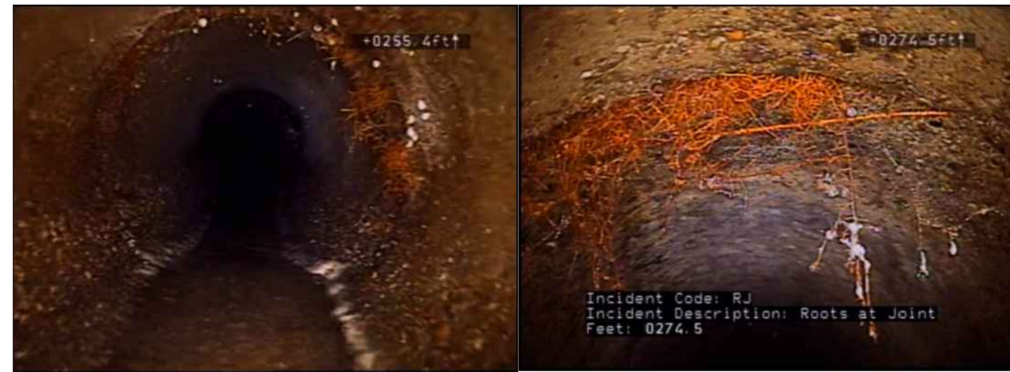
EXISTING MAINLINE CONDITIONS AT SELECT LOCATIONS: MH 72 TO MH 71
