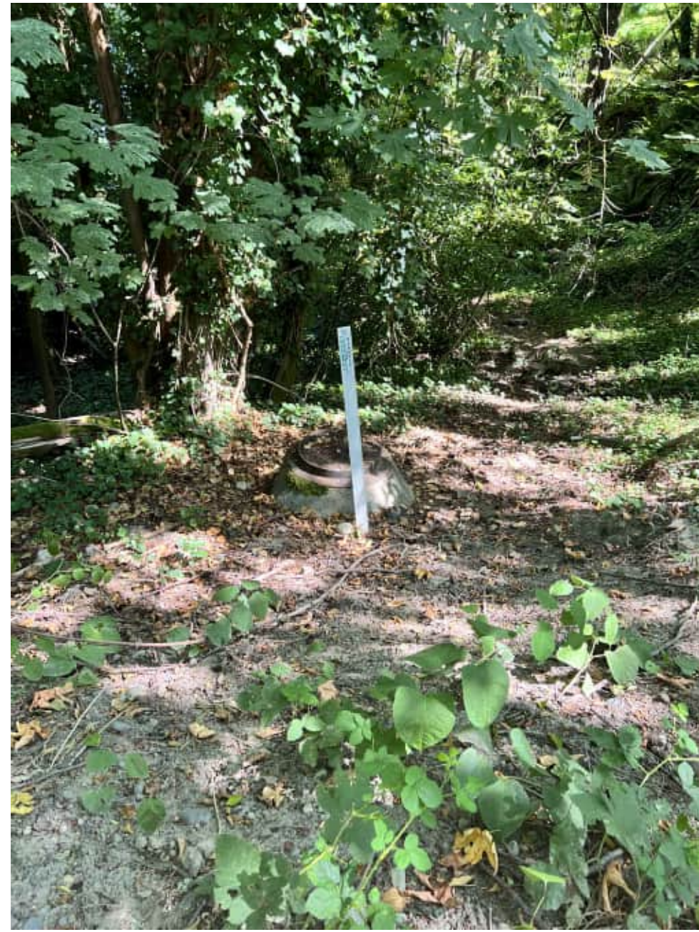
MH LID ACCESS AT SELECT LOCATION: MH 40-6.1
