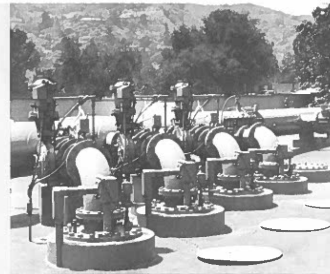
Shown is a submersible booster pump installation in a Municipal Water District in Southern California. The installation includes 3 — 250 HP, 3 — 175 HP, 1 — 125 HP and 1 — 100 HP unit. The pumps were installed in 1957.
