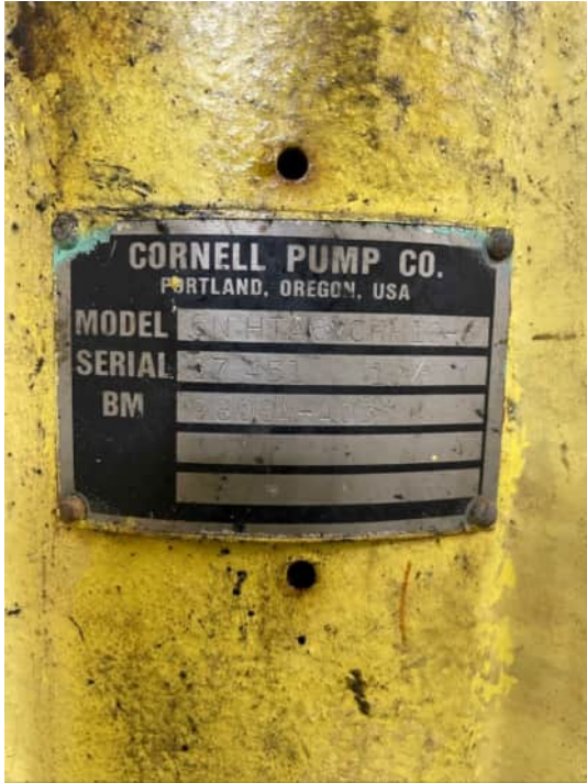
Pump 1 Pump nameplate
