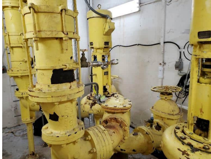
Photo of PS 21 pumps, valves, and fittings on dry well lower level.
