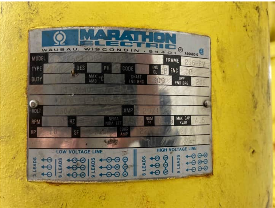
Pump 3 Motor nameplate
