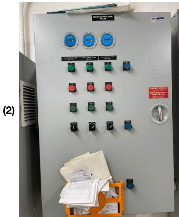
Control Panel Front of the pump control panel
