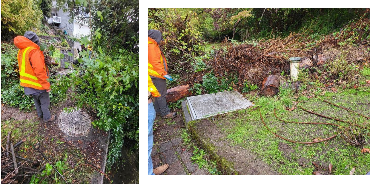
Existing PS 19 site from dock, looking towards dry well access (left). Existing PS 19 site access from the south, looking north (right).
