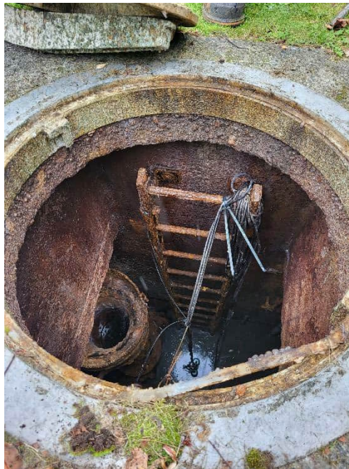
Photo of PS 22 wet well ladder.
