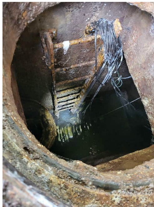
Photo of PS 23 wet well ladder.
