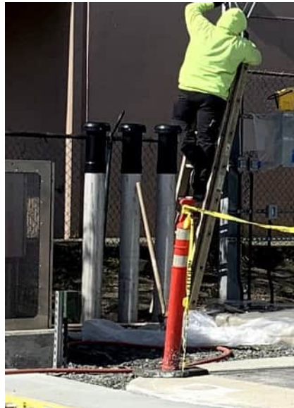
Photo of three in-line carbon filters with exhaust/intake piping at a recently constructed lift station.
