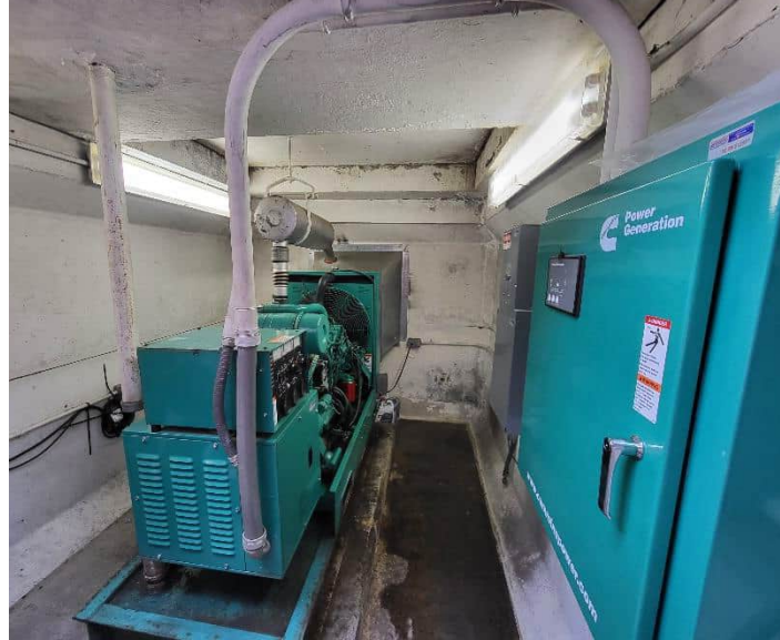
Existing PS 23 below-grade generator room.
