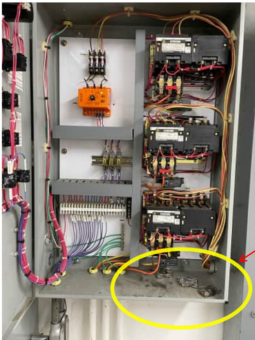
Control Panel Panel interior
