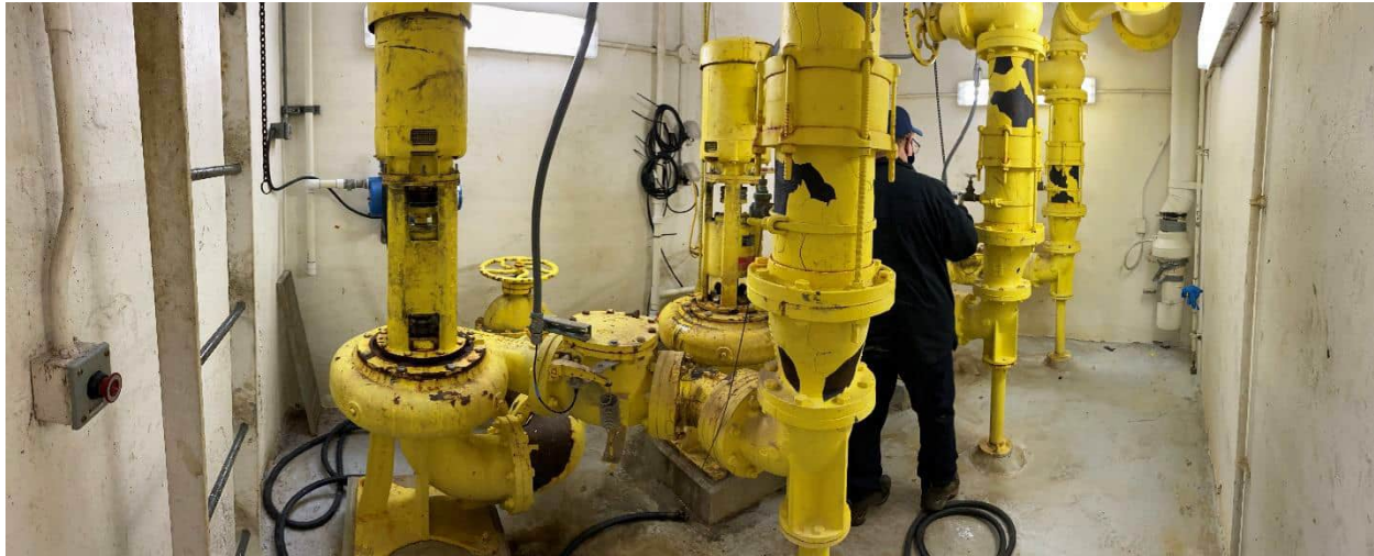
Photo of PS 20 pumps, valves, and fittings on dry well lower level.
