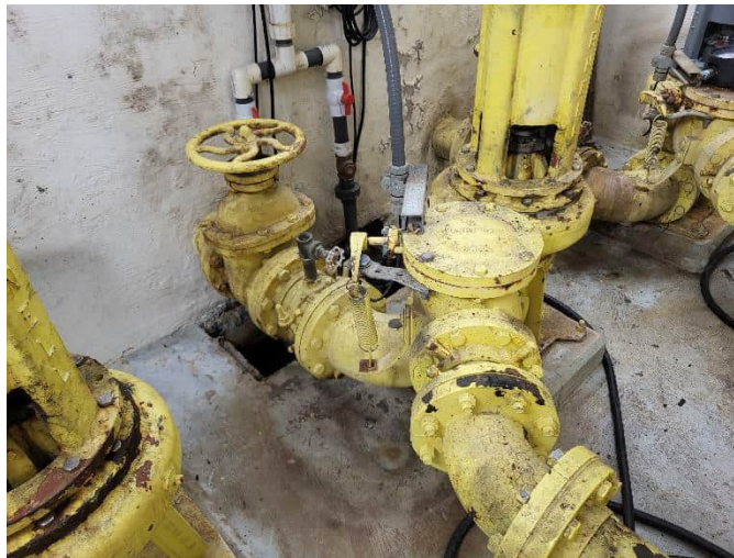
Photo of PS 23 pumps, valves, and fittings on dry well lower level.
