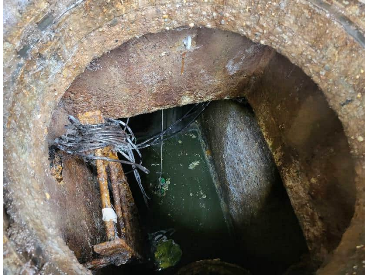
Photo of PS 23 wet well concrete condition.
