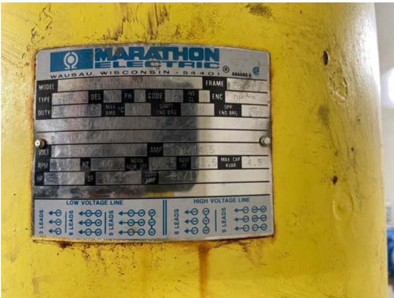
Pump 2 Motor nameplate
