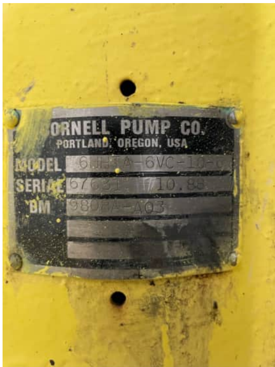
Pump 1 Pump nameplate
