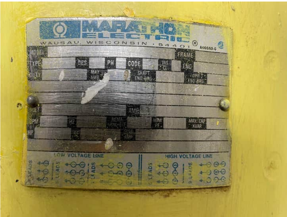
Pump 3 Motor nameplate
