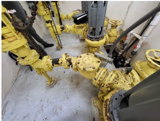
Photo of PS 22 pumps, valves, and fittings on dry well lower level.
