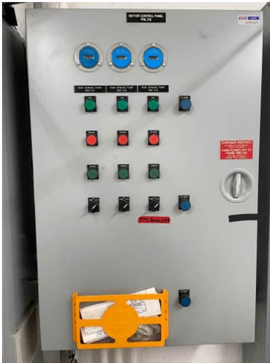
Control Panel Panel front
