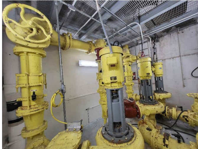
Photo of PS 19 pumps, valves, and fittings on dry well lower level.
