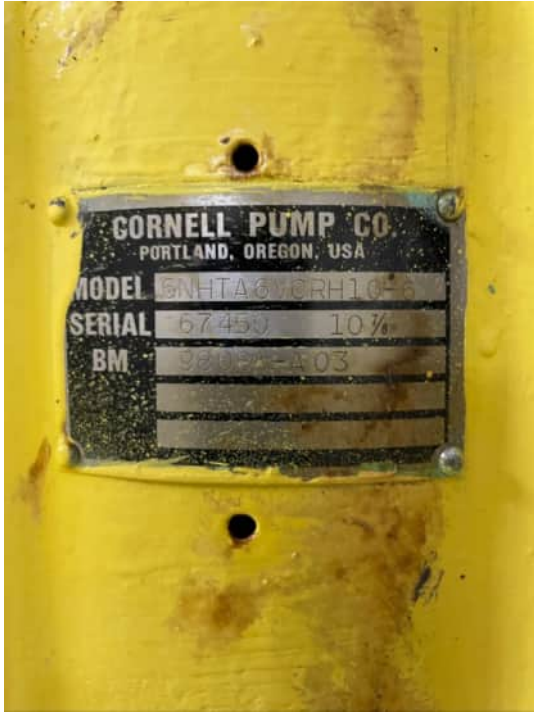
Pump 2 Pump nameplate
