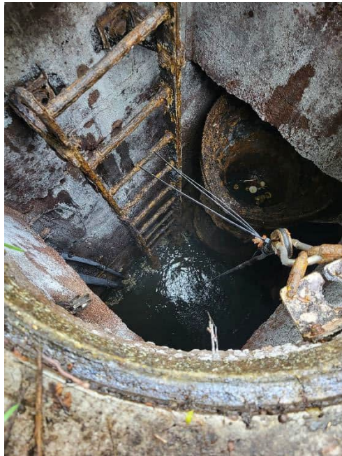
Photo of PS 19 wet well ladder.
