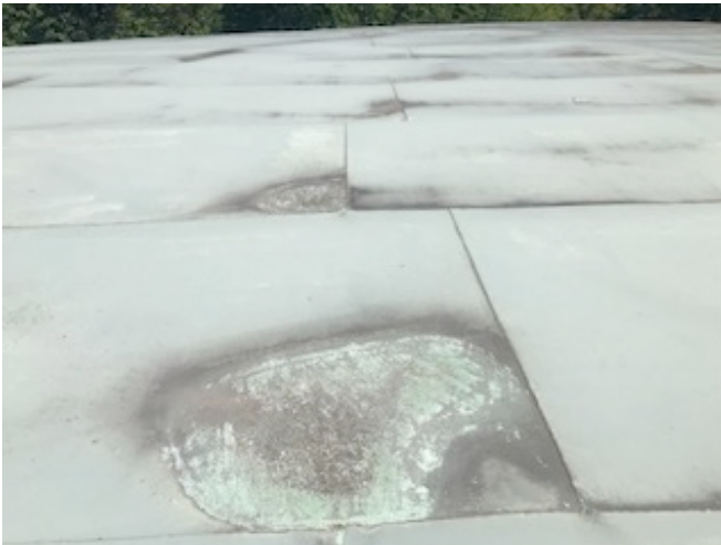
Evidence of ponding water at roof plates, which show a fair amount of inward bowing likely between rafter spacing.
