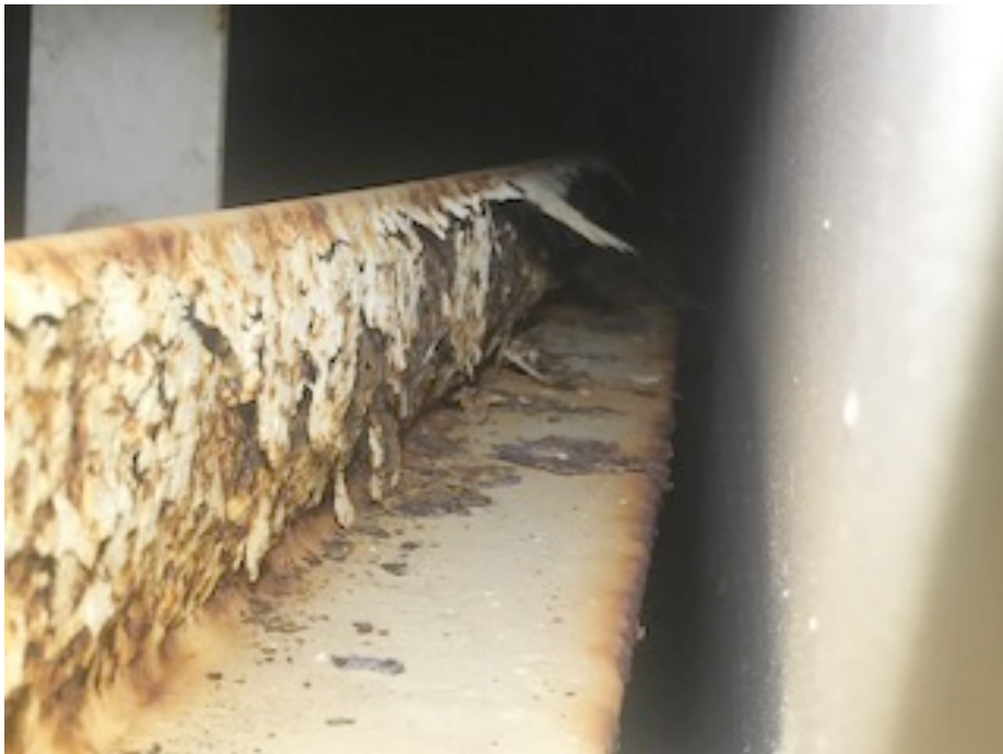
General condition at “backside” of painter’s rail near “knuckle”.
