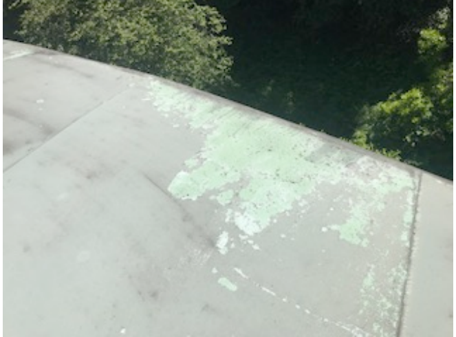
Failed topcoat at roof, minimal corrosion evident.
