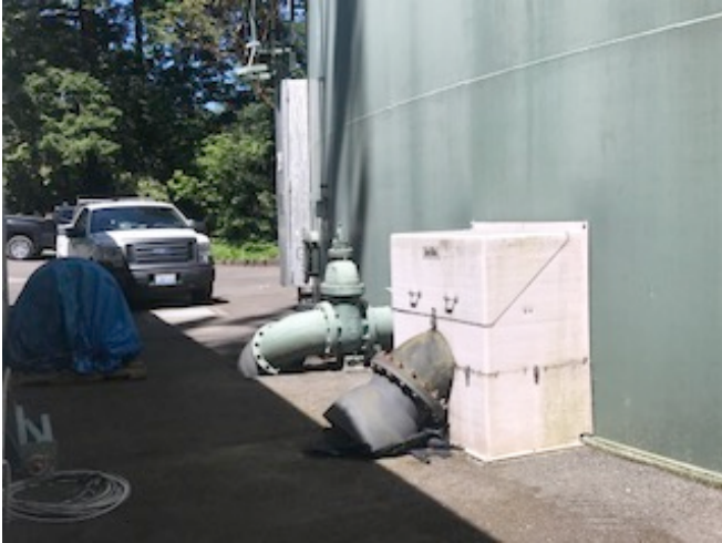
Piping at exterior with shroud.
