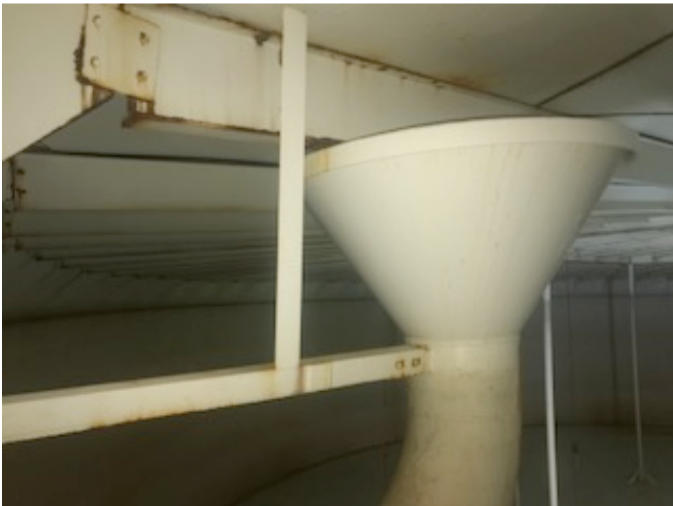
Odd placement of overflow directly below roof rafter, thus making preservation And future coatings work problematic because of access.
