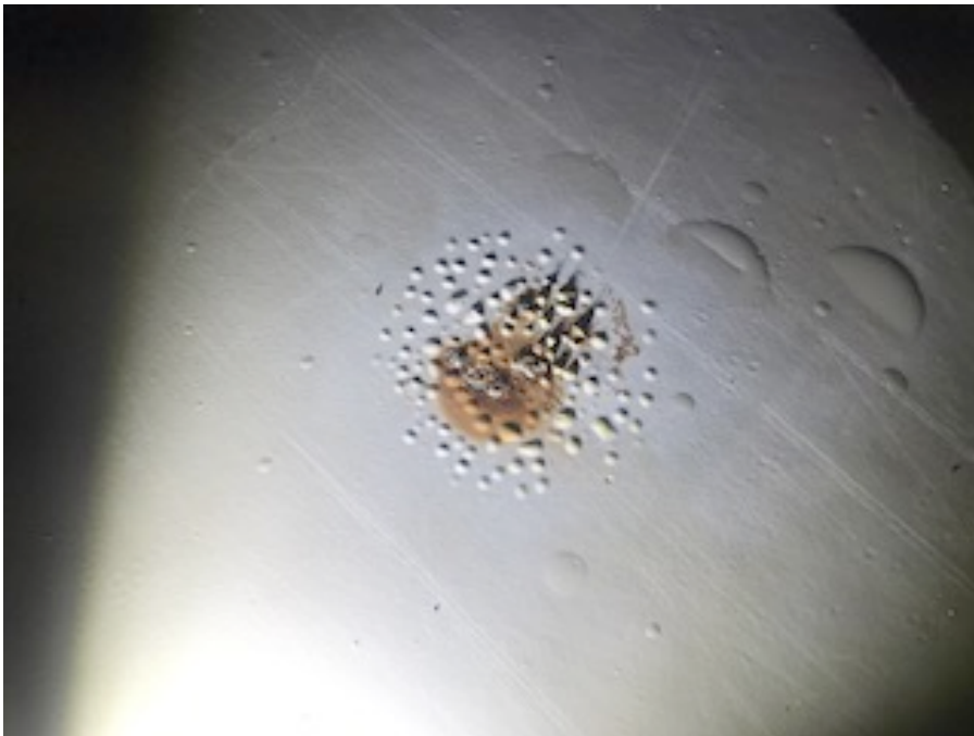
Osmotic blistering at floor – expanding out from pitted steel – isolated corrosion cell.
