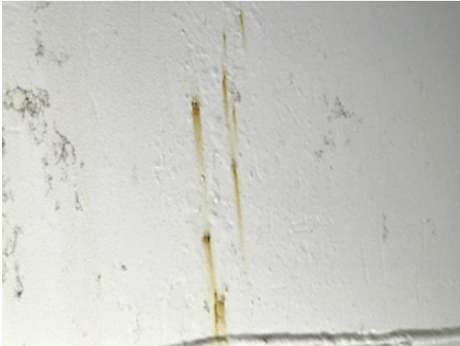
Corrosion noted at shell – upper ring.
