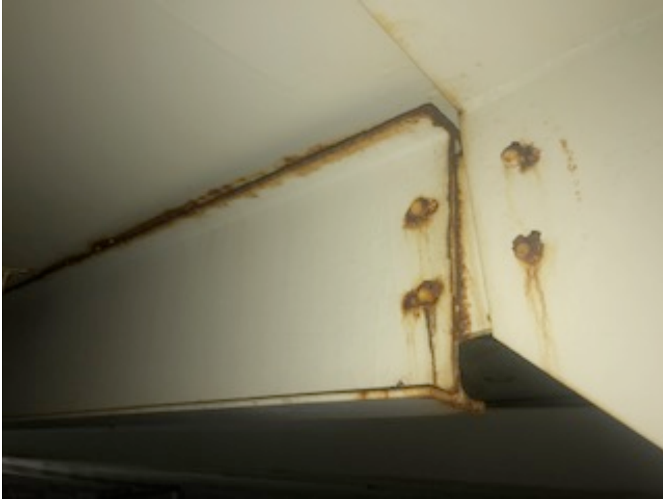
Typical corrosion at edges of rafter, bracket and bolted connection.
