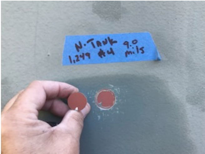
Adhesion test location – cohesive failure of red “lead” Based primer coat.
