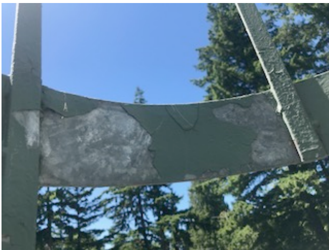
Evidence of HDG underneath failed paint coatings.
