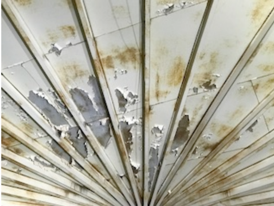
Active coating failure in center ring.
