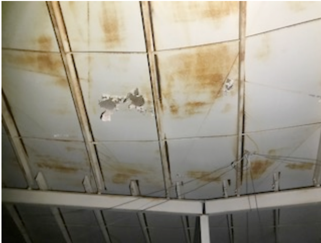
Interior overhead view showing surface corrosion And loosely adhered – failing coating at roof plate.
