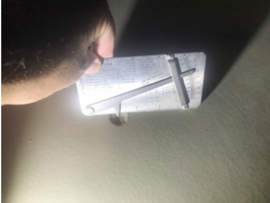
Pitted steel location at floor – approximately 1/8” in depth.
