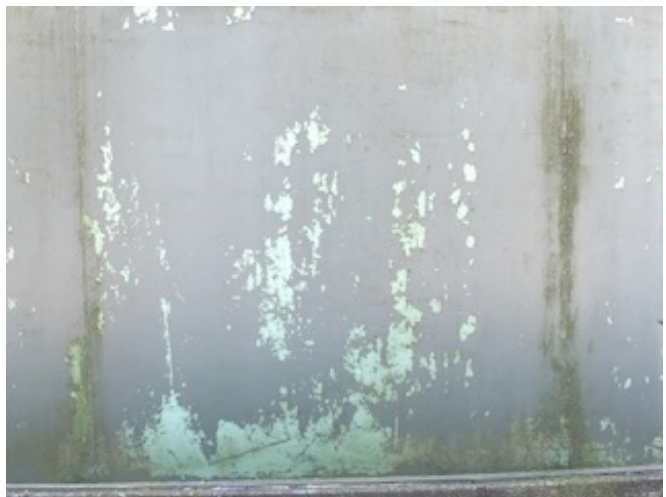
Topcoat failing at shell exterior.
