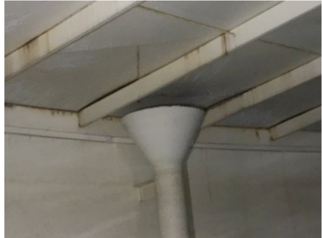
View of overflow near rafters.
