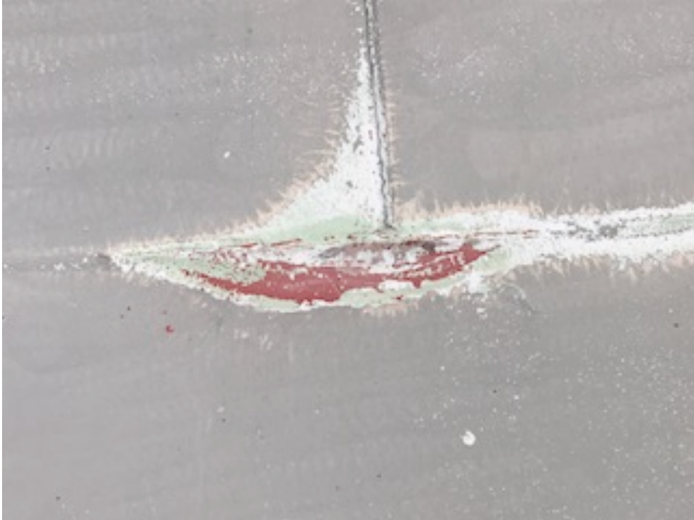
Typical areas at roof with coatings wear – very little corrosion.
