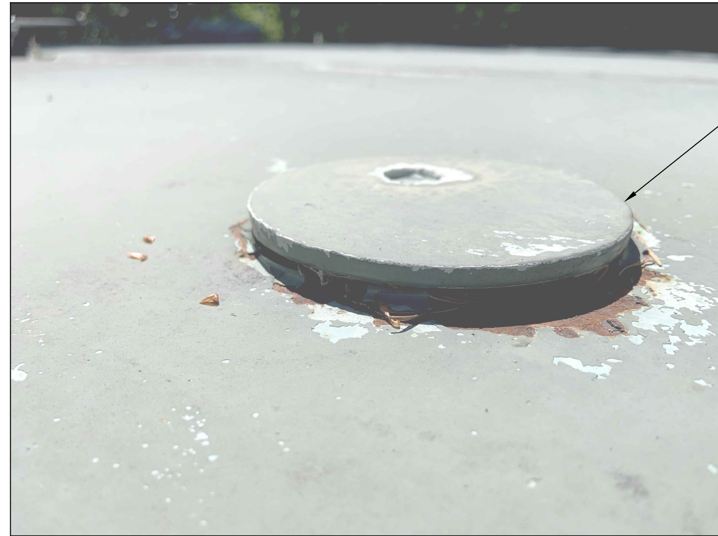
EXISTING ANODE HANDHOLE
